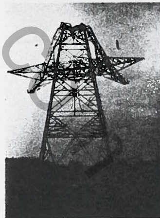
Fig. 7 - Collapsed towers on the Istanbul - Gökçekaya line in a summer incident. Above: transversewise; below: lengthwise.
